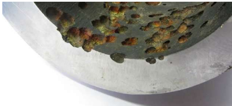
Large Corrosion Pits.
